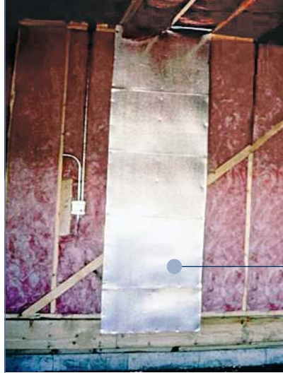
Sheet metal/stud duct
